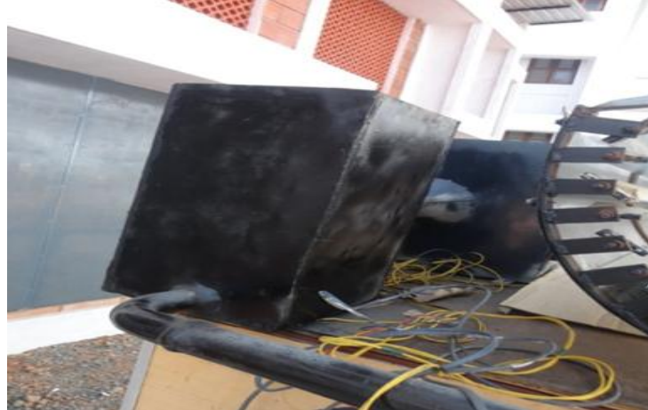
Fig. 6: Fabricated secondary hot water tank
