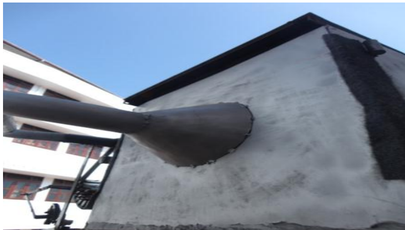
Fig. 4: Inlet duct of the Evaporative chamber
