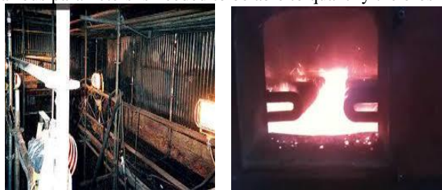
Fig. 1: Corrosion of Bed Coil of Boiler
