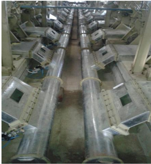
Fig. 3: Non-Continuous Type Pneumatic Conveying Systems
