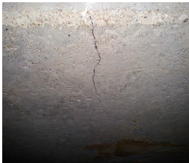
Fig. 8: crack pattern on the edge
